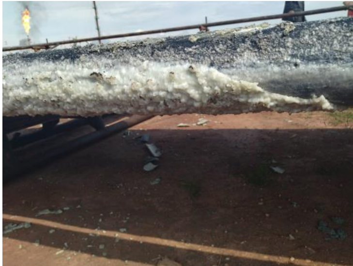
Figure 2. Scale deposits (gypsum) on downhole equipment
